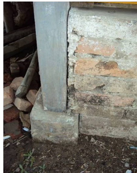
Crack between post and wall
