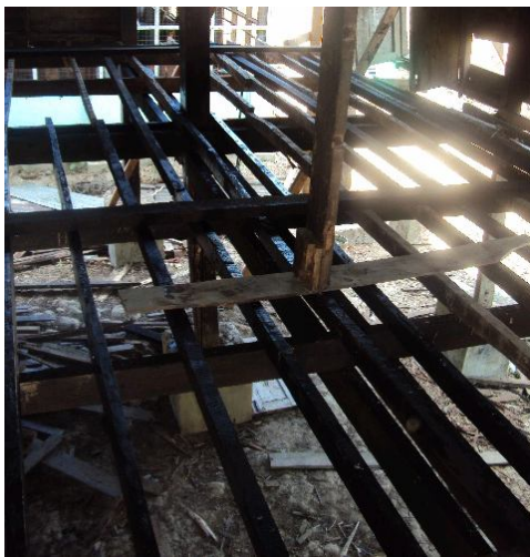
Remove floor panels and replace defects
