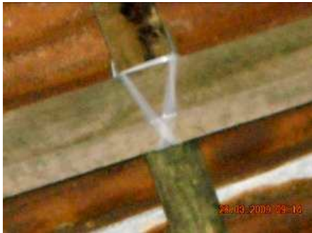
Wire tie between purlin and rafter
