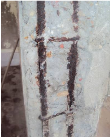
Rusted steel in column
