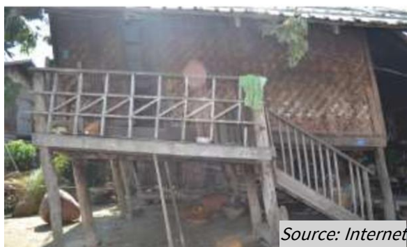
Figure 61: Local damage in some parts of the building
