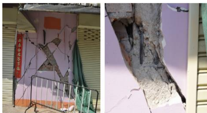
Figure 3: Housing Damages due to Tarlay Earthquake
