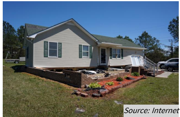
Figure 48: Building off foundation (Severe)
