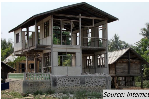
Figure 49: Failure of interior and exterior walls (Moderate)
