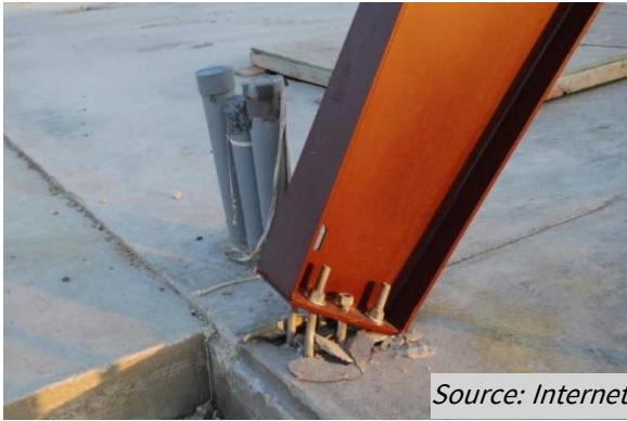
Figure 53: Loose connection (Moderate)
