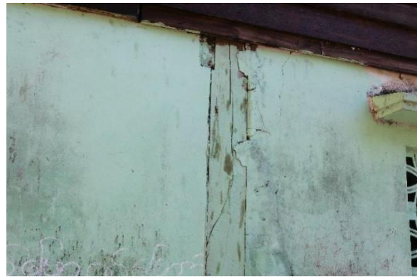
Figure 67: Minor cracks in structural elements
