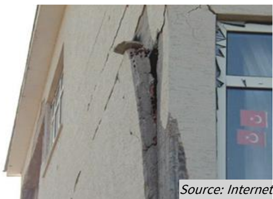
Figure 84: Columns out of plumb or storey leaning
