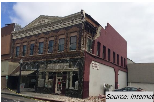
Figure 74: Fall of fairly large pieces of some part of building
