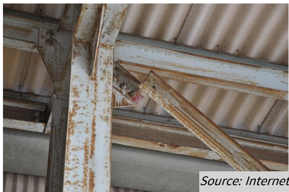
Figure 80: Minor damage in structural members and connections
