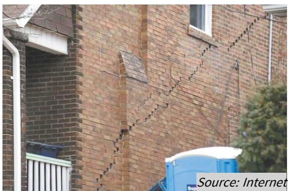
Figure 51: Wall crack in building (Moderate)
