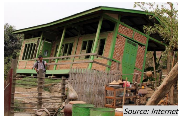
Figure 71: Substantial ground movement, dislocation of the whole building
