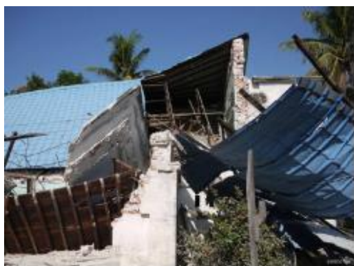
Figure 2: Housing Damages Due to Thabeikyin Earthquake
