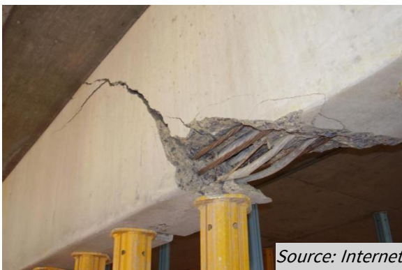
Figure 57: exposure and buckling of reinforcement(severe)
