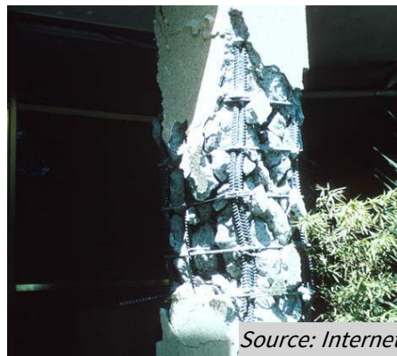
Figure 88: Severe deformation of vertical columns
