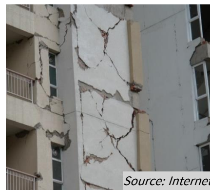
Figure 85: Small cracks in few infill walls or partition walls
