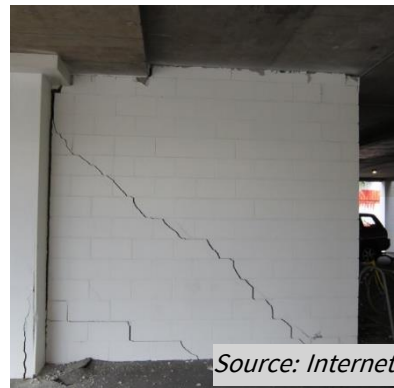
Figure 56: Large diagonal in partition or infill walls (Moderate)
