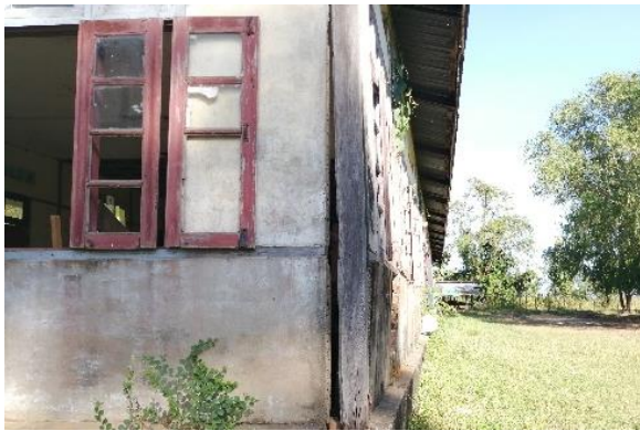
Figure 66: Slight separation of walls from timber post
