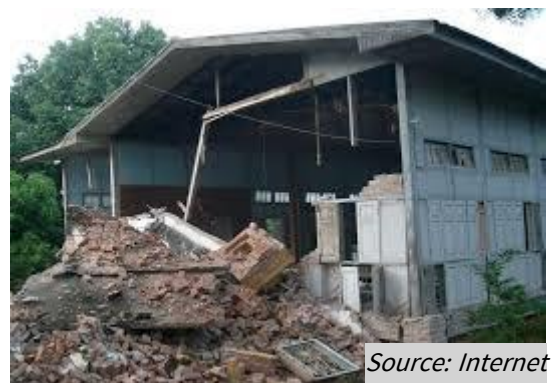
Figure 50: Partial collapse (Severe)
