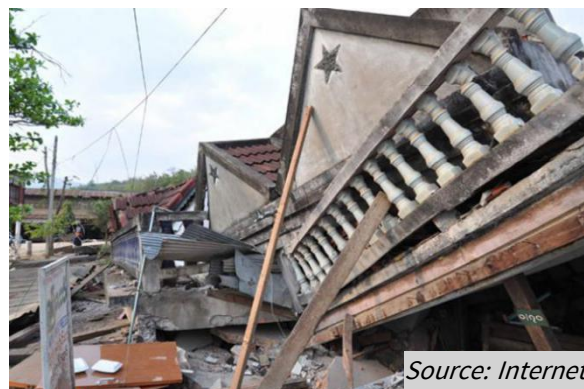
Figure 78: Substantial ground movement and leaning of the whole building
