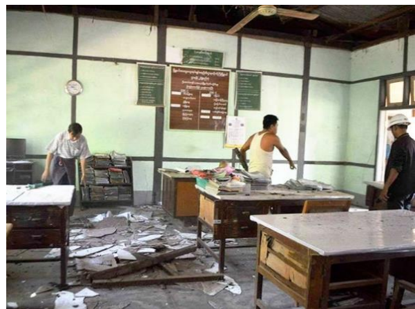
Figure 9: Post Earthquake Assessment after Taiky Earthquake
