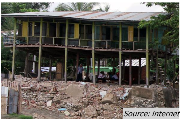
Figure 70: Failure of interior and/or exterior walls
